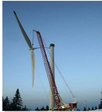
Lifting a rotor at the RES Canada SNEEC site in Gaspé, Québec in December 2009 - A fine balance!
